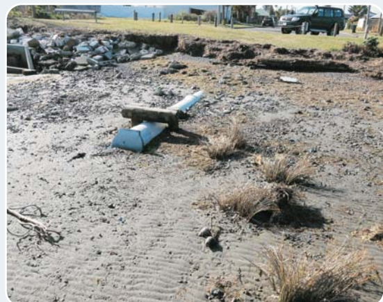
Stressed stormwater infrastructure: The erosion scarp gives an indication of how far the coast has retreated since the construction of the outlet. The image also illustrates how low the roading and housing infrastructure is (notice the ad hoc riprap infill). Photo: Ian Wright, Christchurch City Council.
