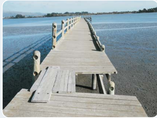
Boardwalk adjacent to the South New Brighton Community Centre. The gap in the boardwalk has been bridged where the structure has been pulled apart by liquefaction-induced lateral spreading. The entire structure has sunk, warped and been pulled apart by more than 2 metres by this earthquake-induced process. Photo: Ian Wright, Christchurch City Council.
