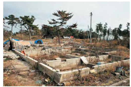
Figure 4: Concrete slabs and foundation walls are the only remnants of most timber-framed buildings that were in the tsunami’s path. Before being swept away, the timber frame was anchored to a concrete base using the steel bolts visible in this picture as protruding black sticks (Dec. 2011). Photo: C Gomez.
