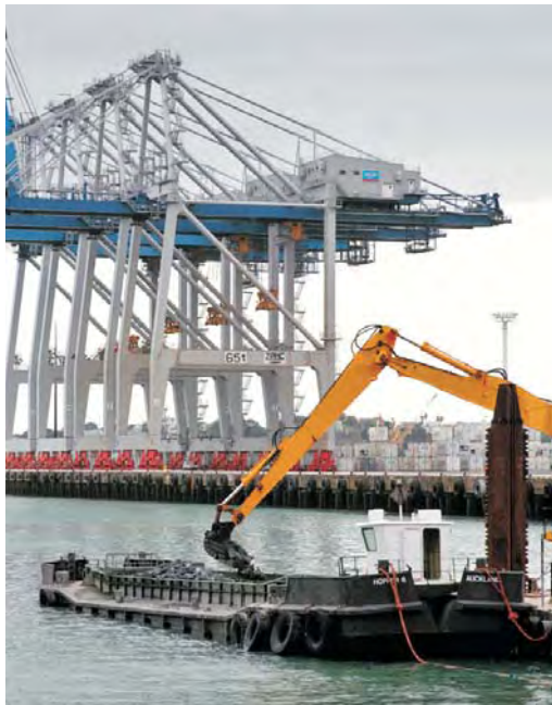
Deepening the outer berth at Fergusson Container Terminal. Photo: Ports of Auckland.
