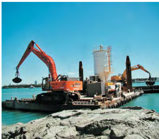
The Fergusson Deepening project will deepen the berth from -12.5 m to -13.5 m at lowest of low tides. Photo: Ports of Auckland.
