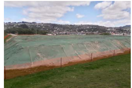
Dunedin City Council's sand stockpiling at Kettle Park. A spray-on polymer has been applied to the sand surface to minimise wind-blown erosion (Photo: Tom Simons-Smith).
