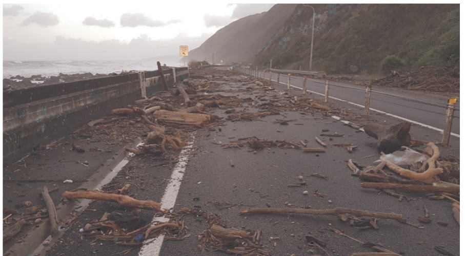
Figure 1: Debris from the sea that overtopped the Coast Road (SH1) north of Wellington after ex-cyclone Gita (Photo: WSP Opus).
