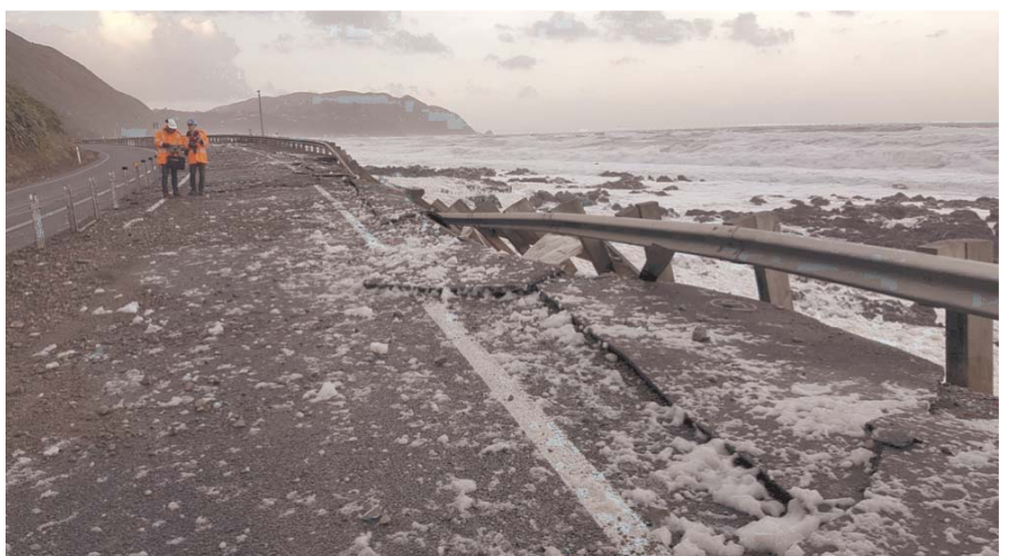
Figure 2: Damage to road infrastructure on the Coast Road (SH1) north of Wellington after ex-cyclone Gita (Photo: WSP Opus).
