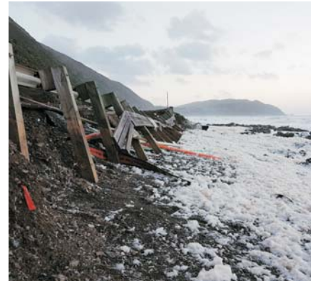
Damage to SH1 north of Wellington after ex-cyclone Gita (Photo: WSP Opus).
