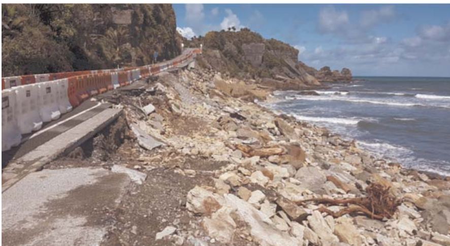
Figure 5: Punakaiki section (SH6) damaged after ex-tropical cyclone Fehi (Photo: WSP Opus).
