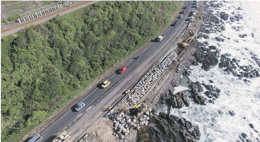
Figure 3: Drone footage of the Coast Road (SH1) during emergency works – only one lane is operative (Photo: WSP Opus).
