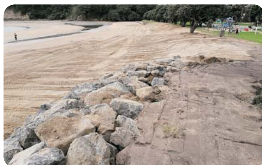
(R) Figure 10: Reconstructed rock revetment in front of toilet block (Photo: Matthew McNeil, Auckland Council).
