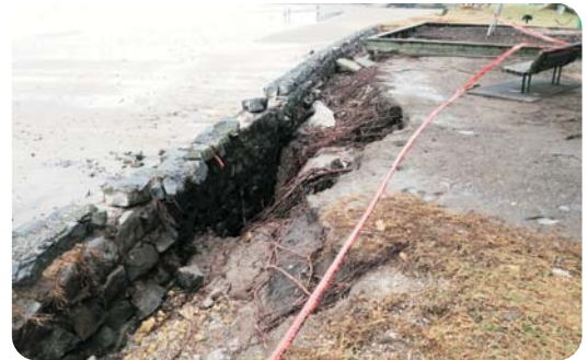
(Below) Figure 6: Mairangi Bay, 5 January 2018, scour behind seawall (Photo: Matthew McNeil, Auckland Council).
