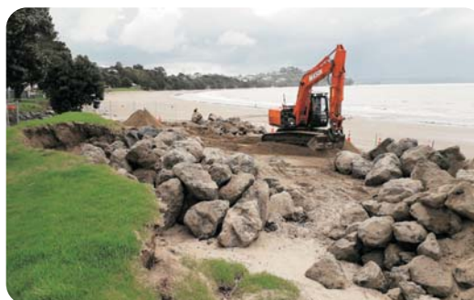
(L) Figure 7: Stanmore Bay, outflanked rock armouring and eroded reserve edge, 5 January 2018 (Photos: Paul Klinac, Auckland Council).
