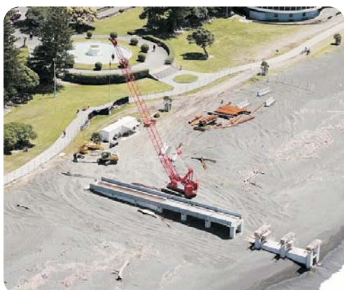
Construction for Napier's stormwater outfall and viewing platform on the Marine Parade Reserve began in August 2015. Above photos: Napier City Council.
